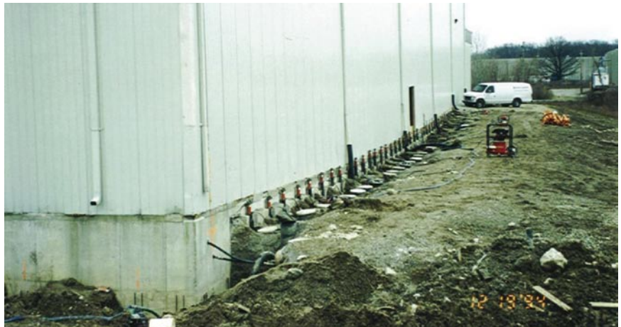
The photo above shows the right side being carefully and gently lifted. Note the hydraulic rams on each pier.
