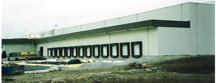
This is a view of the front of the structure. The loading dock shown here had settled 8 inches. Some areas at the right side of this building suffered settlement in excess of 22 inches!
